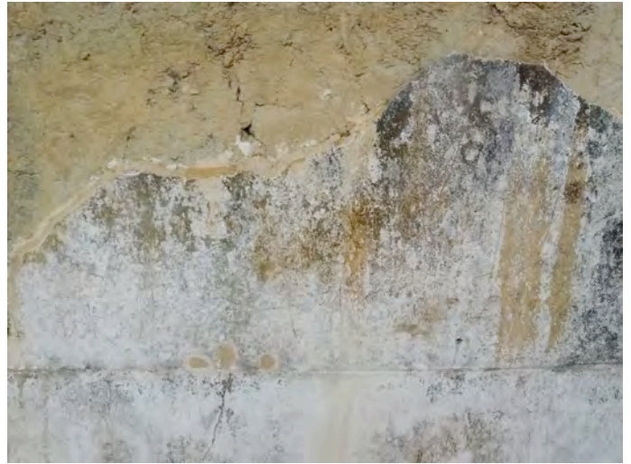
Figure 8. One of the 3 test areas after grouting of the delaminated plaster. Judging from percussion testing after curing the grout distributed well and re-established adhesion between plaster and substrate (Photo: Gesa Schwantes).
