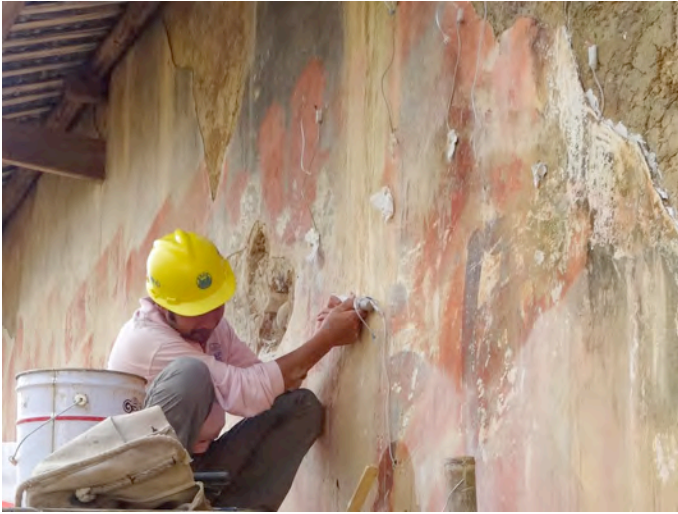
Figure 1. Application of water based NHL grout for reattachment of clay plaster at Liu's Family Ancestor Hall, Jinggangshan, Jiangxi. Water from pre-wetting and grout is transporting to the surface. (Photo: Dai Shi Bing)
