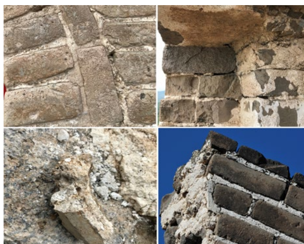
Figure 4: Pointing and bedding mortars (above calcium lime with hydraulic components, below dolomitic lime). Source: Dai Shibing
