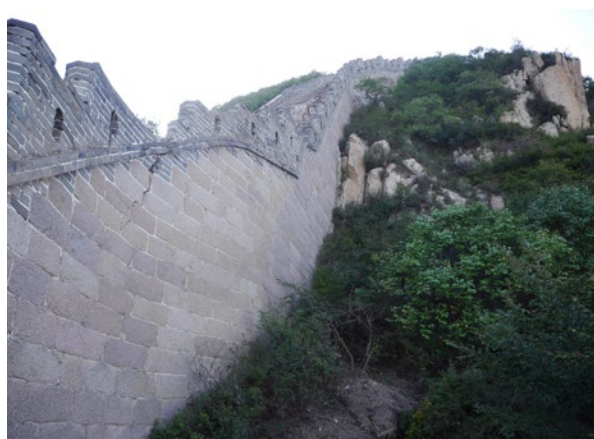
Figure 2: Wall surface from granite and bricks with white dolomitic lime mortar showing cracks and delamination, Source: Dai Shibing
