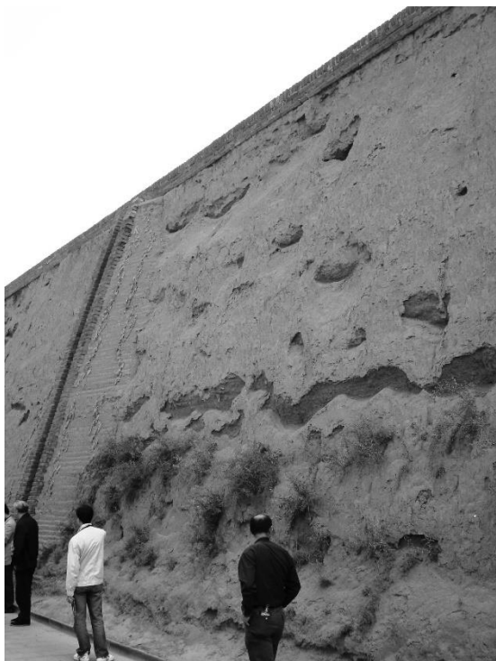
Figure 2 Erosion of earth and repeated maintenance (photo taken in 2006)
