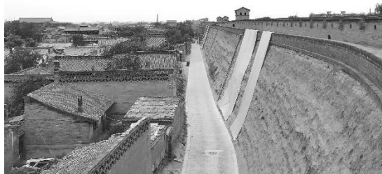
Figure 1 Internal rammed earth finishing of the Historic Wall of Pingyao (photo taken in 2018). The areas covered by plastic sheets are in danger to collapse.
