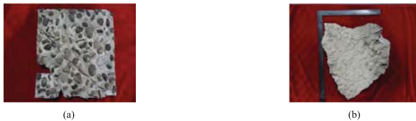
Fig. 2. (a) Dash pebble uncovered with coating (D1), (b) dash pebble covered with later coating (D2)
