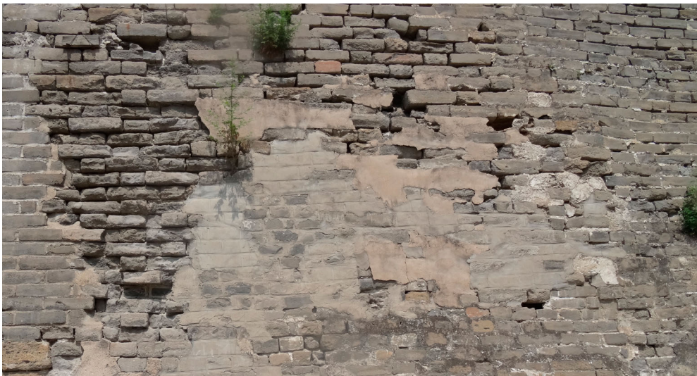
Figure 11. Brick work of the Great Wall from Ming Dynasty was restored many times with cement mortars, which have caused more deterioration than conservation (photo by Hu Zhan-Yong).
