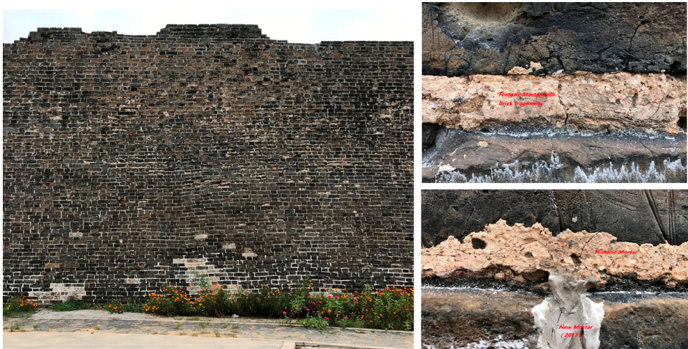
Figure 2. Thick bedded historic lime mortars (light beige-ocker coloured) with inclusion built between 1369 and 1375. Modified air lime (light grey coloured) was used for the restoration of the brick wall in 2017 using, which is not compatible neither in colour, texture, nor in the physi-chemical properties.
