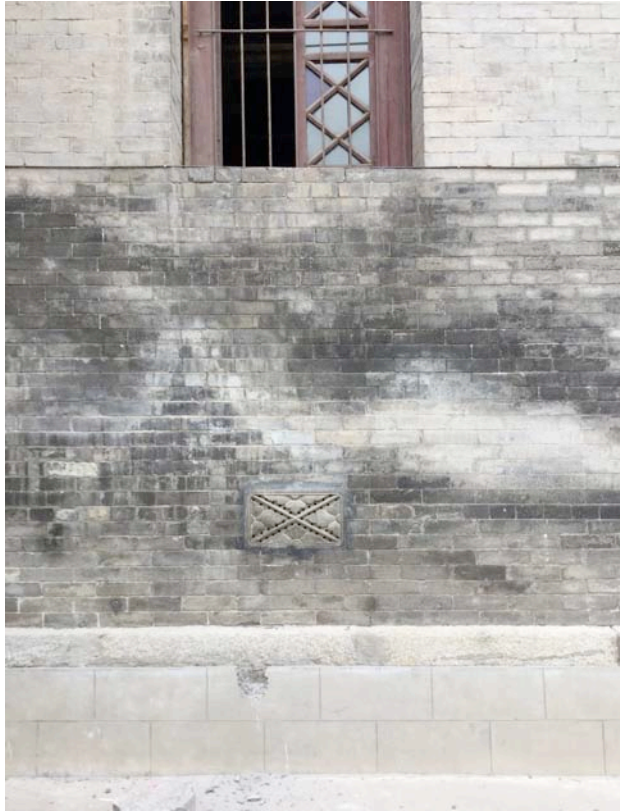
Bild 1: Cement plaster used for repairs of a brick wall at St. Francis Cathedral, built 1716 in Xian. The repair work at the wall base as well as repairs to the damaged bricks were carried out with incorrect materials (cement) causing damage to the original façade.
