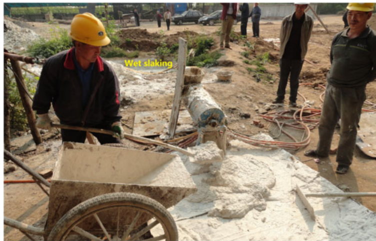
Figure 3 Wet slaking and preparation of lime with hemp fibers during restoration works in southern Shanxi 2012.
